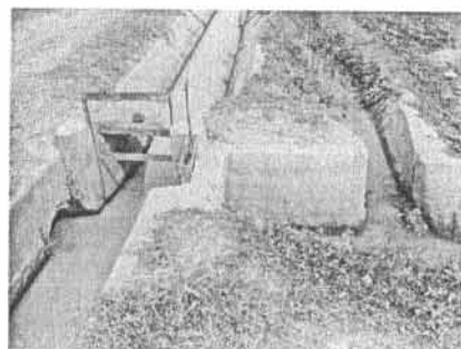
Photo 6: absence de vannette
