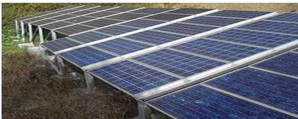
Plaque solaire photovoltaïque
