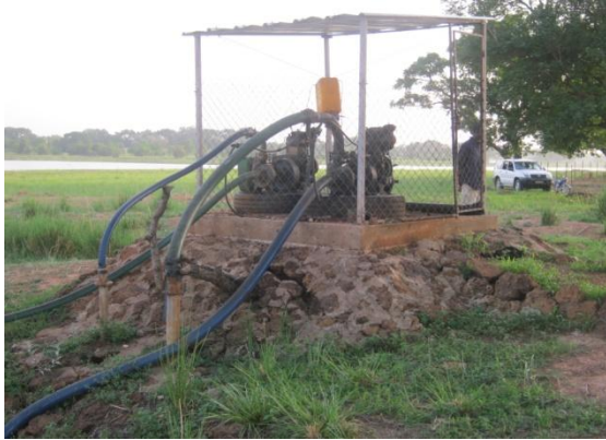
Station de pompage (Mars 2012)
