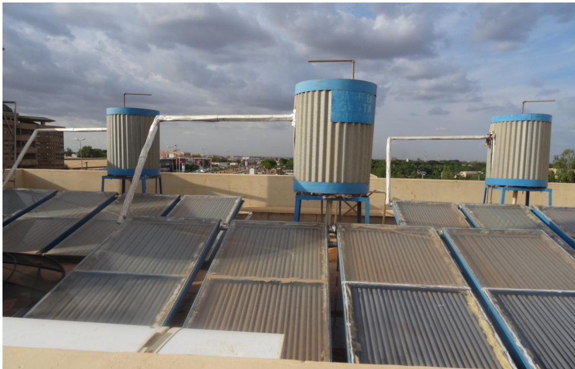
Figure 8: Installation de chauffe eau solaire de la Residence Alice.
