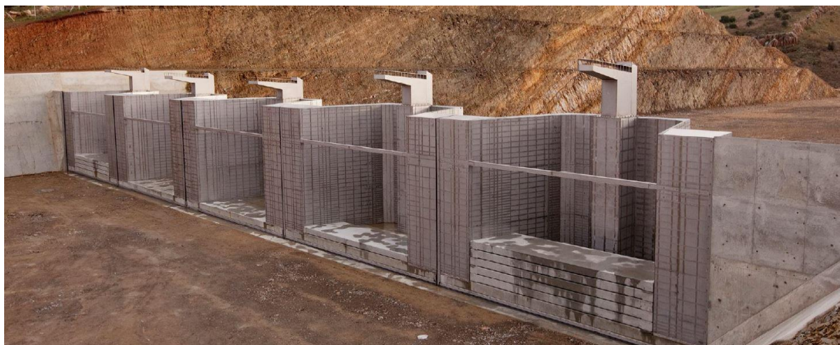
Figure 2: Image hausse fusible _source Hydroplus
