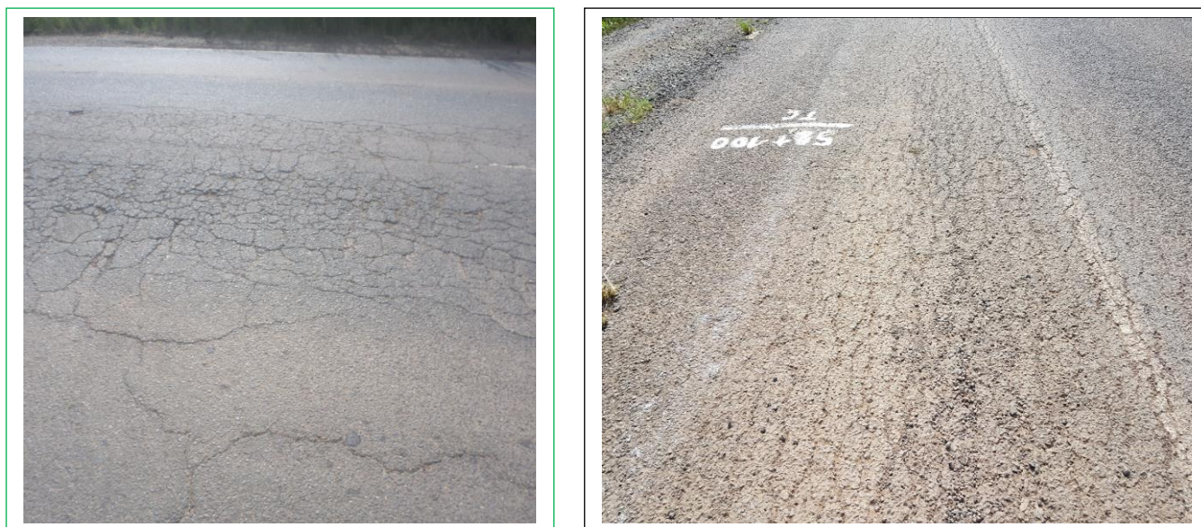
Figure 4: images illustratives des fissures
