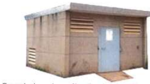
Figure 6: Poste en Cabine (H59) [1]
