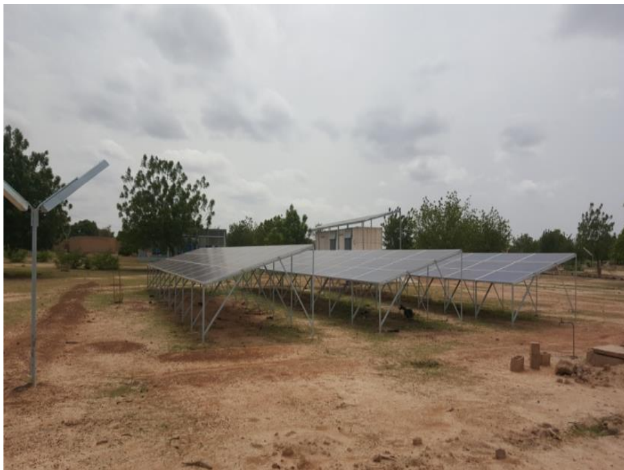
Figure 13 : Champ Photovoltaïque de 30 kWc
