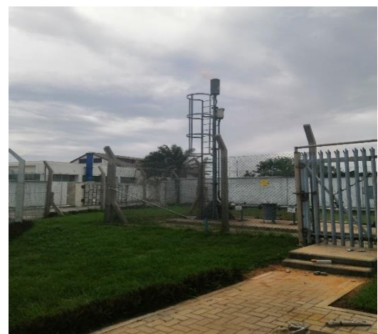
Figure 3-J: Biogas Flaring Unit
