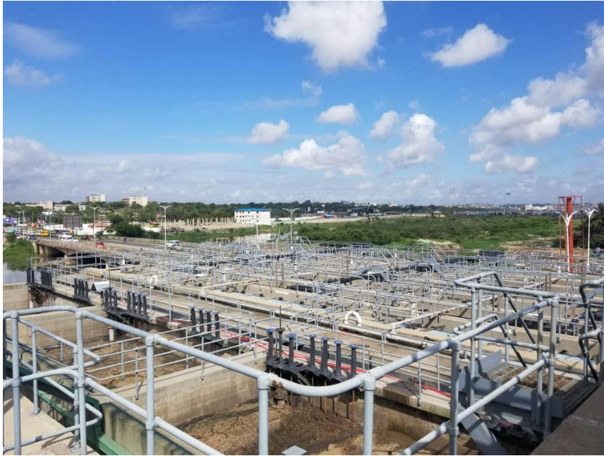
Figure 3-F: The UASB Reactors and Sludge Thickeners
