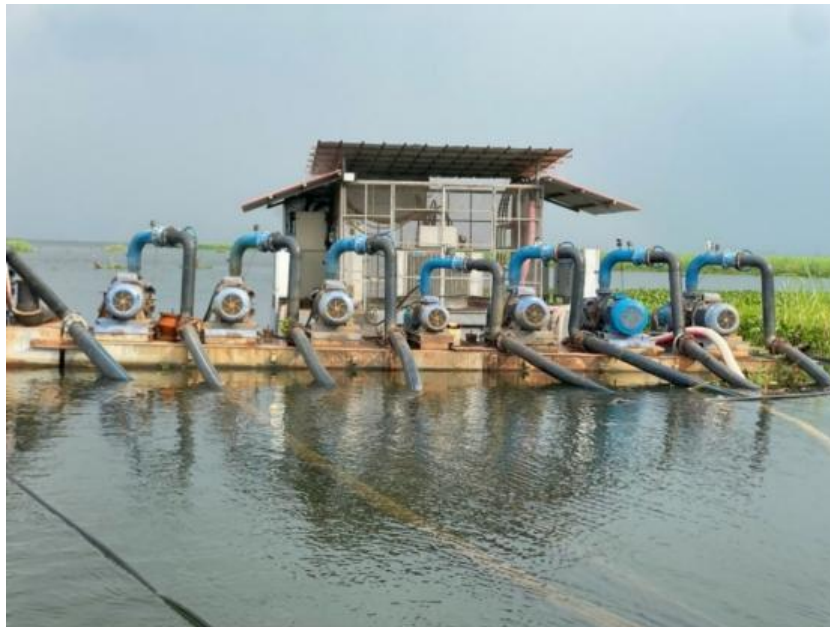
Figure 7: Station de pompage Ahondo II
