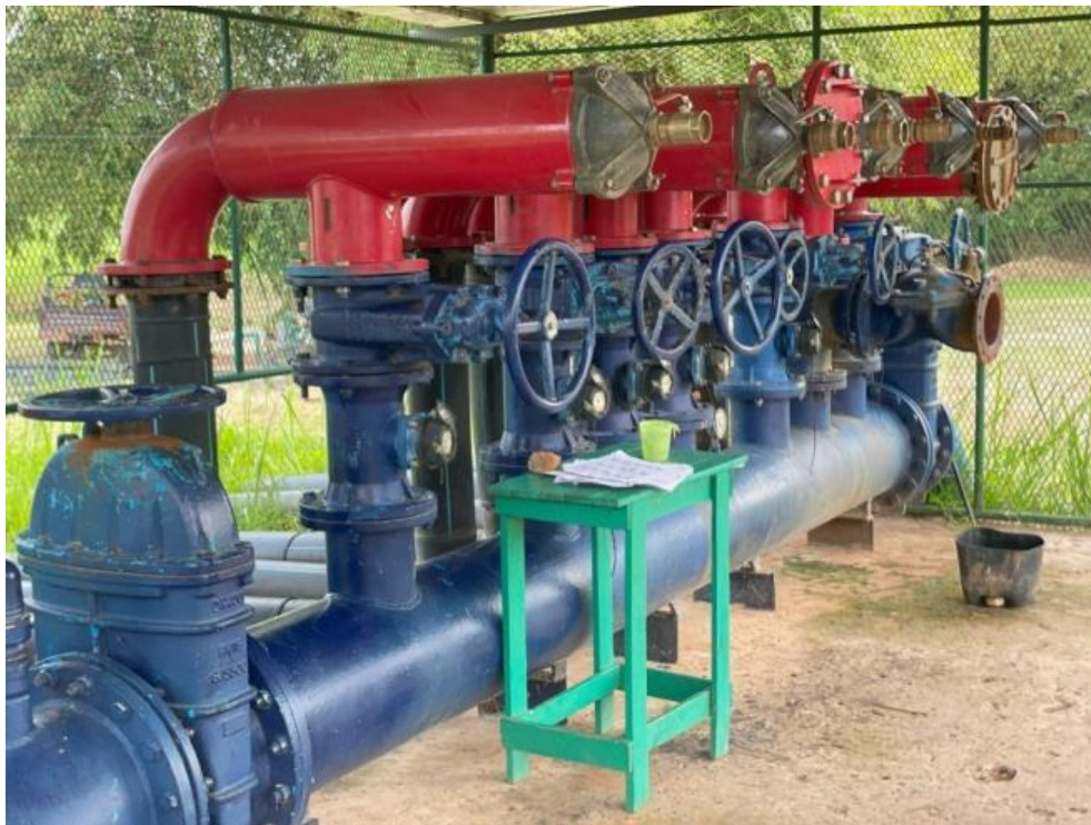
Figure 8: Station de filtration Ahondo II
