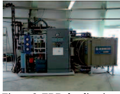
Figure 8. EDR desalination plant.
