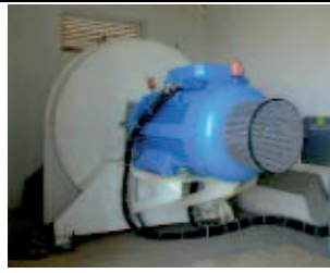
Figure 5. 100 kVA Synchronous machine coupled to flywheel.
