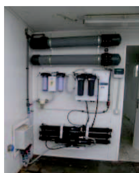
Figure 26. View of the MORENA SWRO unit.
