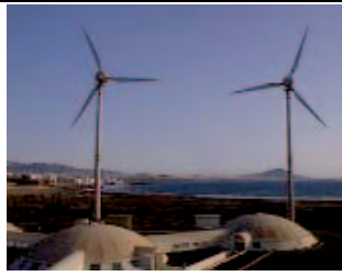
Figure 4. 2 x 225 kW off grid wind farm.
